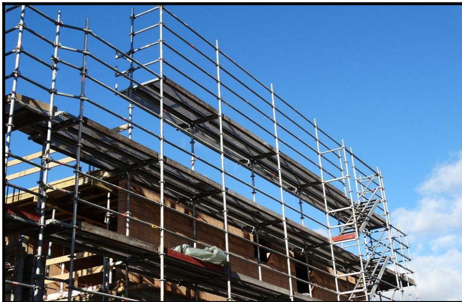
Photo courtesy of OSHA.GOV
